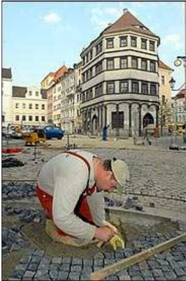
Matthias Rietschel for The New York Times HISTORY IN THE REMAKING A worker lays bricks in the Untermarkt.
